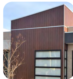
COMPLETE: After 3 coats the colour of the panels is restored. Maintain the stain at regular intervals, according to stain supplier recommendations.
